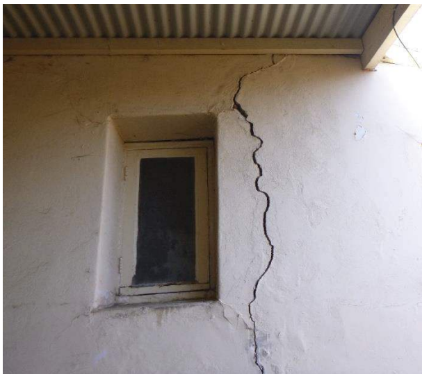
Major cracking between main house and lean-to
