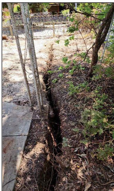
8.3 mtr long by 600 mm deep trench to driveway and car port edge.
