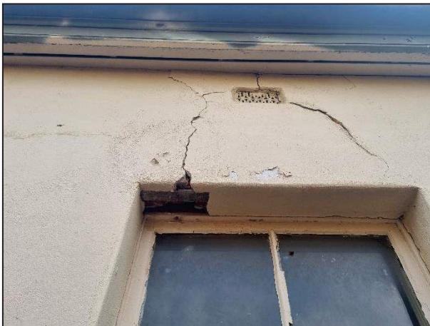
Photo 6 – Structural cracking over lintel on southern external wall
