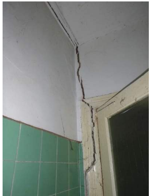
Major cracking – Bathroom
