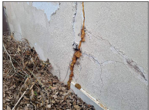
Photo 9 – Structural cracking to southern external wall with evidence of prior gap filling (inadequate)
