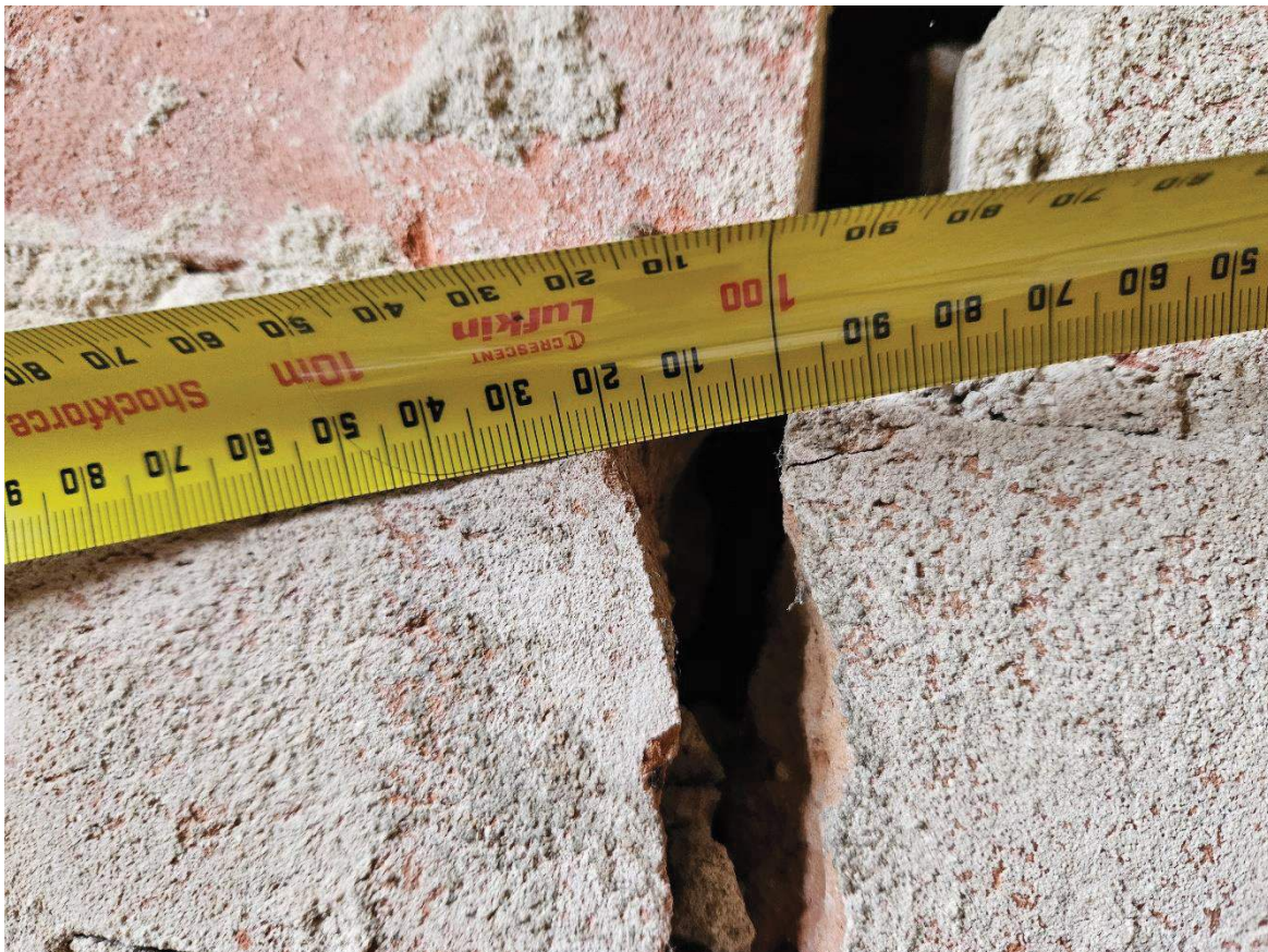
Photo 2 – Close up of crackingshown in Photo 1
