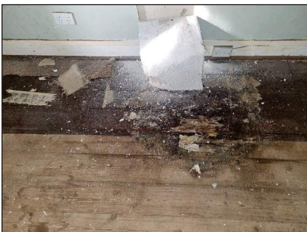
Photo 12 – Moisture damage to timber floorboards due to roof leak above
