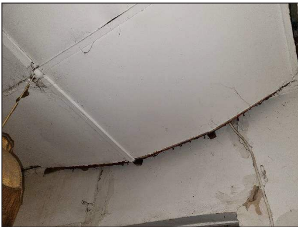
Photo 10 – Collapsed ceiling to rear addition
