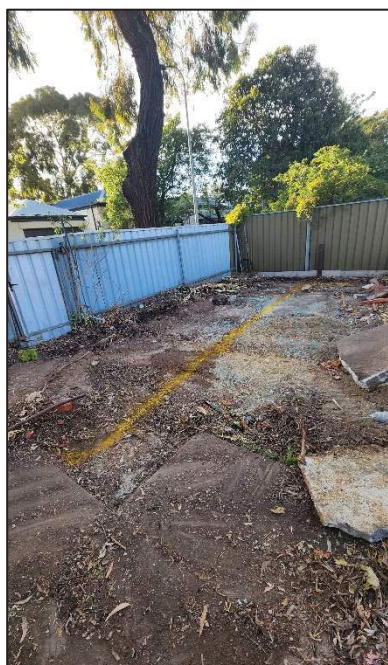
Discovery mark out 2.5 mtrs off eastern boundary after garage and slab demolished.
