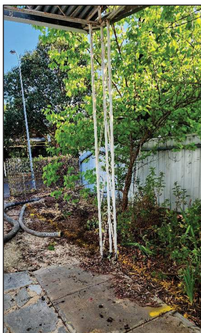
Discovery mark out 2.5 mtrs off eastern boundary. Small tree likely responsible for roots 13-15.
