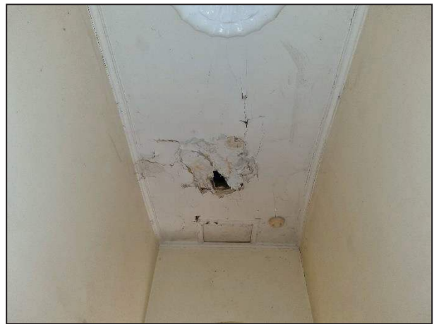
Photo 11 – Collapsed plaster ceiling due to roof leak
