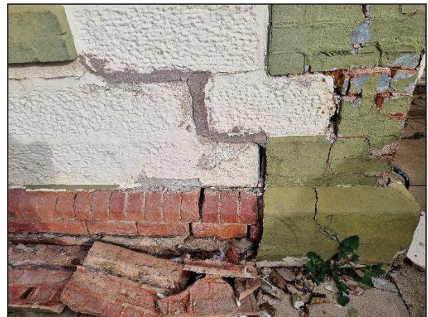
Photo 7 – Structural cracking to northern eastern external walls with evidence of prior crack filling
