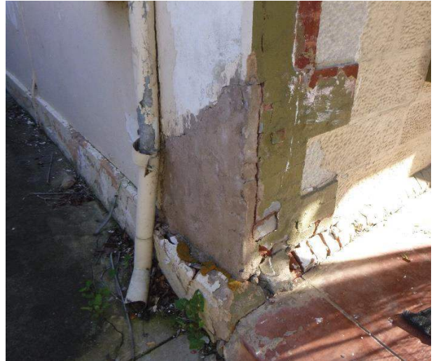
Severe deterioration in south-eastern corner
