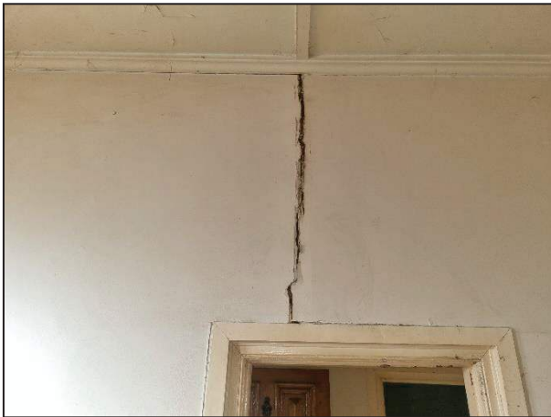
Photo 2 – Severe structural cracking to internal wall
