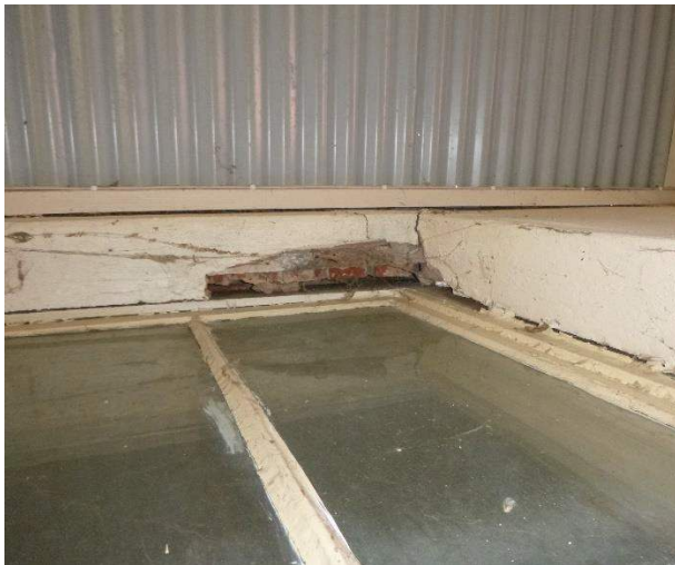
Severe deterioration of brickwork above bedroom 3 window
