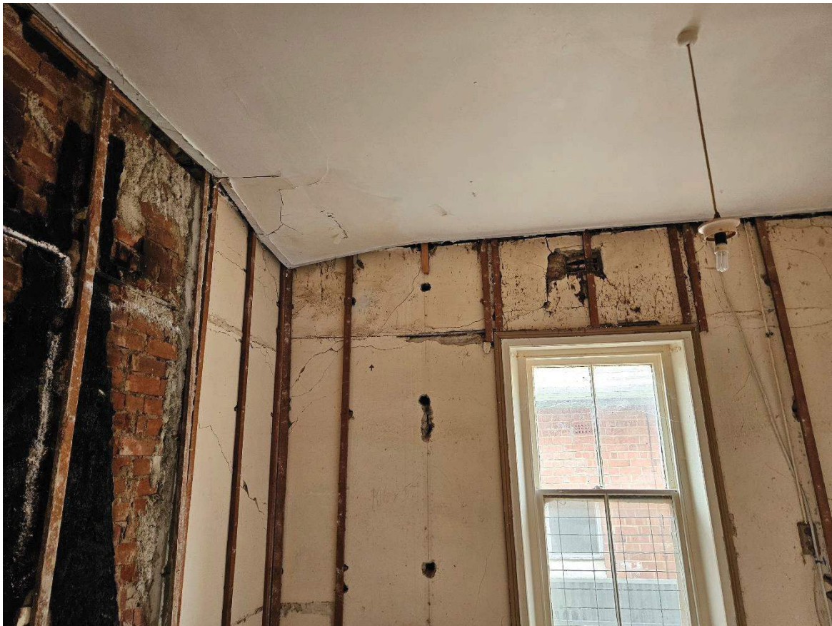
Photo 13 – Living room's ceiling has detached from frame in south-eastern corner
