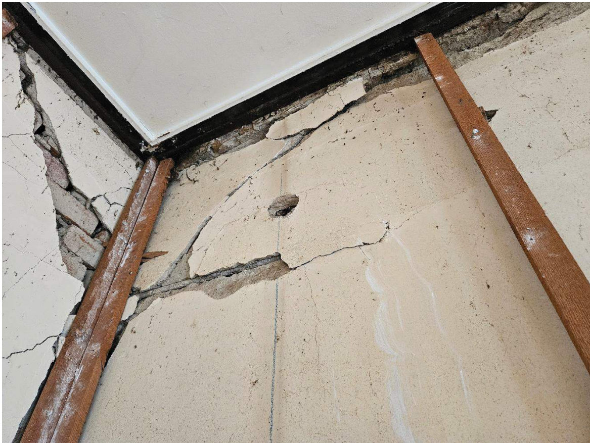
Photo 7 – Tie-rod chased into northern wall of Bed 1, distortion to walls and deterioration of plaster
