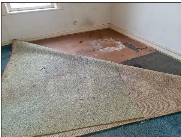
Photo 4 – Dropped floor in south-western room
