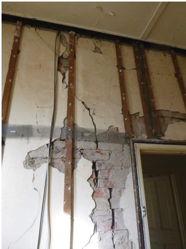
Major cracking – Lounge
