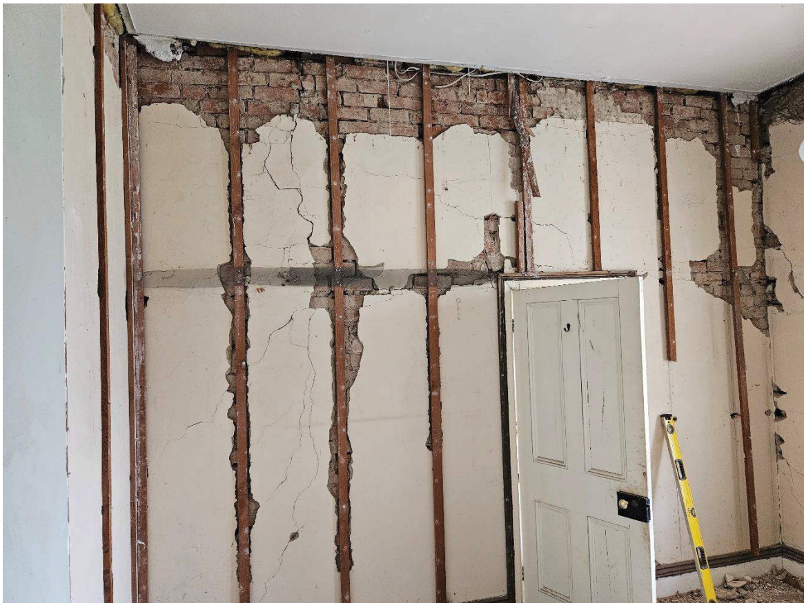
Photo 10 – Overall view of Bed 2's northern wall showing condition of plaster
