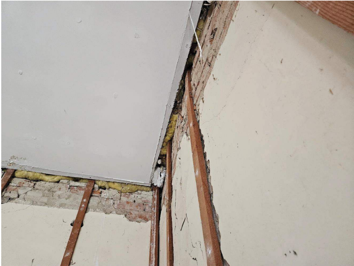
Photo 9 – View of northern Bed 2 wall showing out of plane movement
