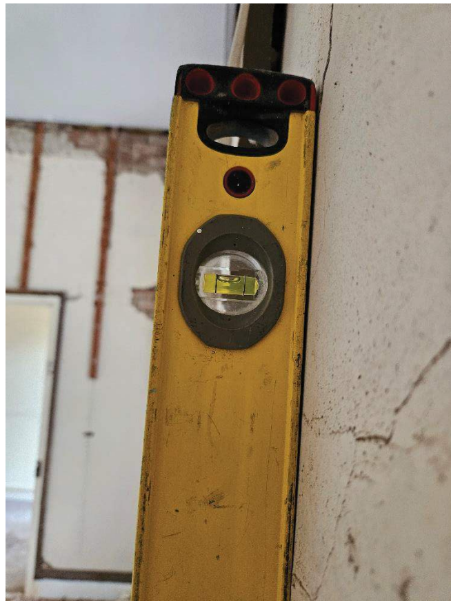
Photo 12 – Rotation of Bed 2's eastern wall consistent with long-term settlement towards east
