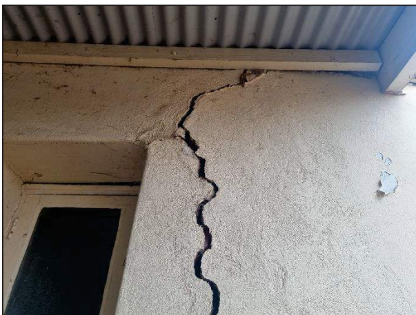
Photo 8 – Structural cracking (Category 4 – Severe) to northern external wall
