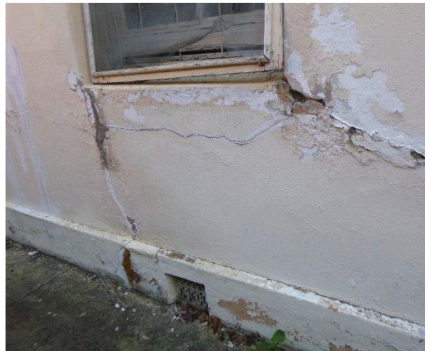
Severe cracking around bedroom 2 window
