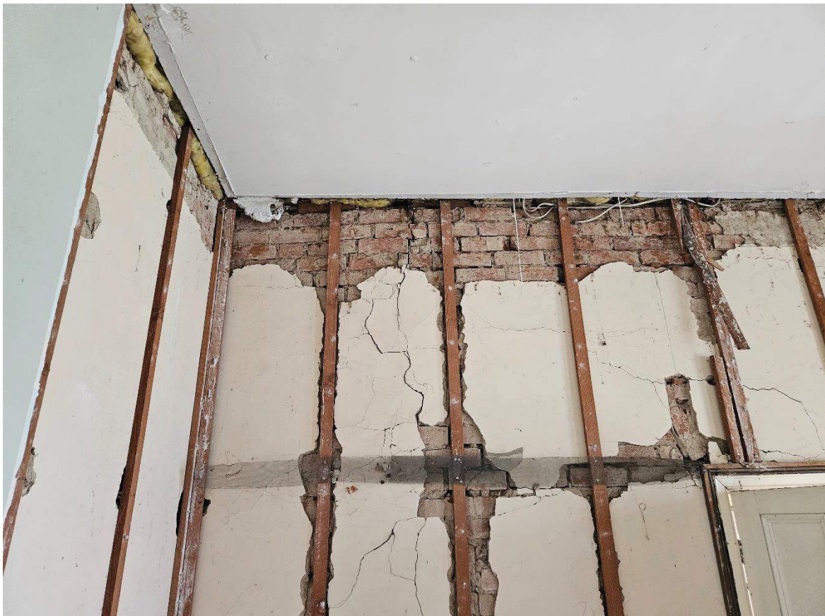
Photo 8 – Bed 2's northern wall, brickwork to top half of wall requires reconstruction
