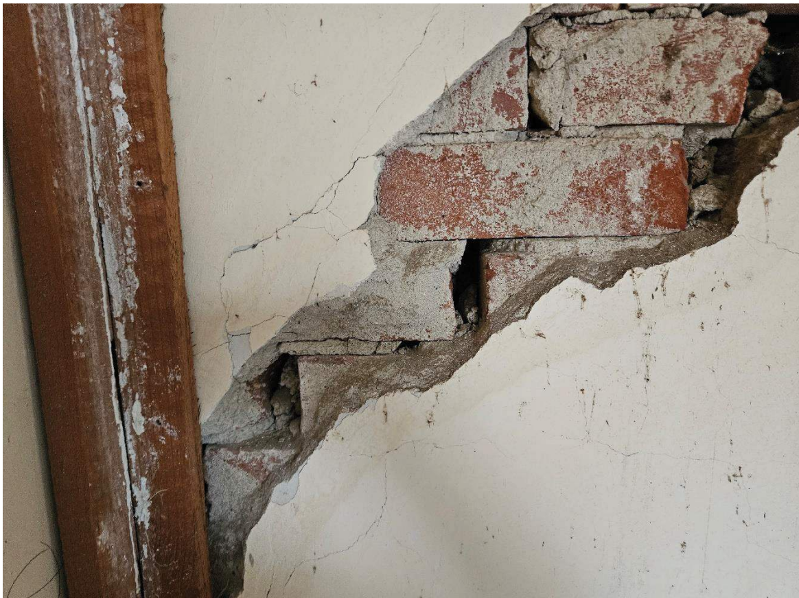
Photo 18 – Cracking to Living room's northern wall
