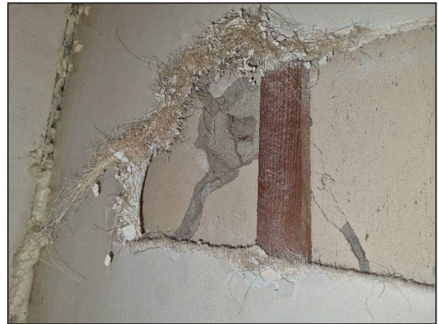
Photo 3 – Cracking to external wall concealed behind fibrous plaster cladding
