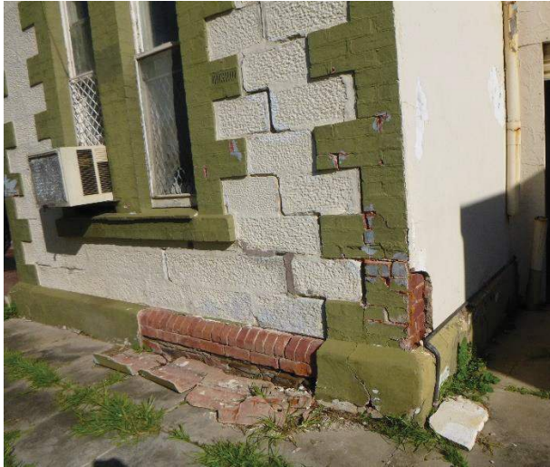
Major cracking and deterioration in north-eastern corner
