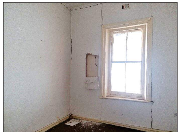
Photo 5 – Typical cracking to internal plasterboard claddings
