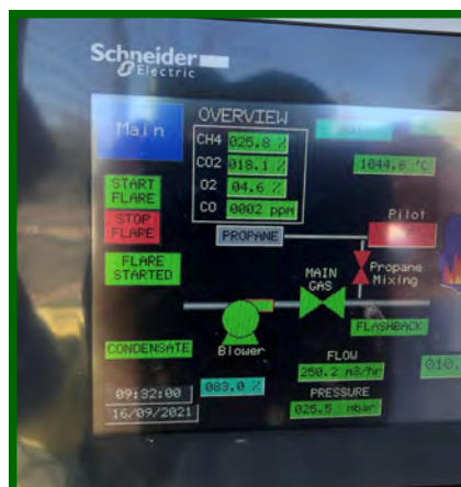
Control panel of flare operating
